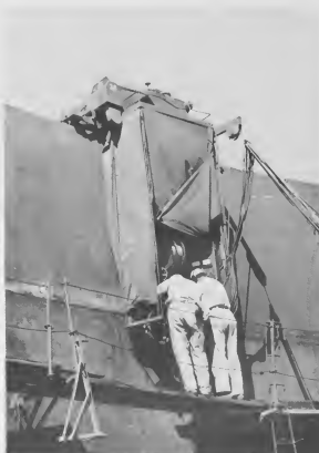
ONE OF the fascinating devices used in building the tanks is the automatic welding machine that looks like a voting booth, runs like a trolley and welds horizontal seams. Faster and straighter than a crew of men. UN DI e aparatonan fascinante usá den construcion di tankinan ta e mashine automatico di welding, cu ta parece manera un urna electoral, ta corre manera un trolley y ta weldo seams horizontal.
